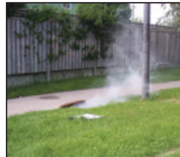
Smoke exiting a sewer manhole
