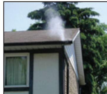
Smoke exiting a downspout
