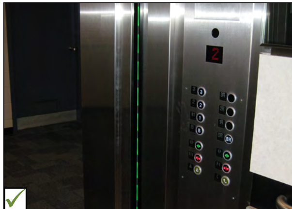
Elevator sensor door and floor registration buttons.
